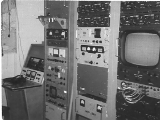
Yet another configuration - Nems Clarke TM receiver and spectrum display in the center rack. Telemetry demodulation and display gear in the right hand rack.
